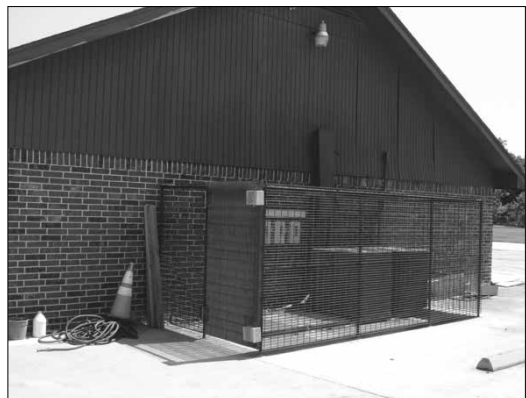
Example: This photograph illustrates AC units protected by a steel cage and security lighting.
