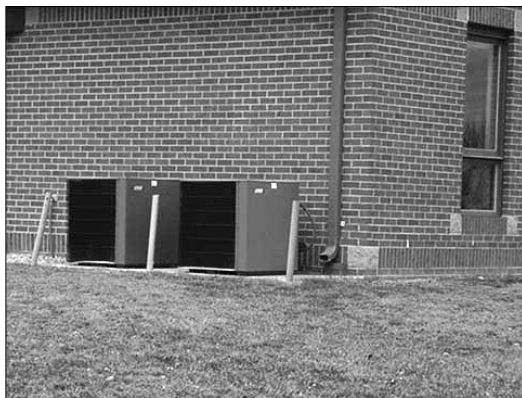
Example: This photograph illustrates AC units located at the back of the building creating an easy target for theft.
