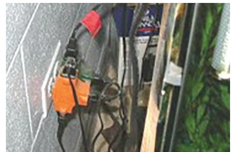
This image represents inadequate wiring. This practice should not be permitted.
