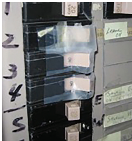
Image above shows breakers taped in the "ON" position. This practice should never be done.
