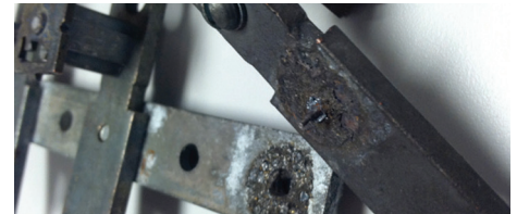
This is a failed, high-resistance, busbar connection inside a 200 ampere Stab-Lok panel. The arced-away steel screw holds the copper bar in the foreground to the aluminum bar in the background.
