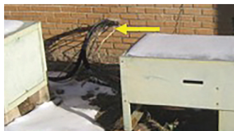
Image above shows an inadequate wiring set up for the central air conditioning units. Electrical is wired directly to the A/C condensing units, without a safety disconnect.
