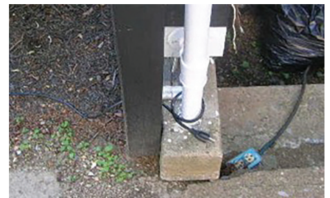
This image shows an outdoor wiring installation that is not a GFCI protected receptacle.
