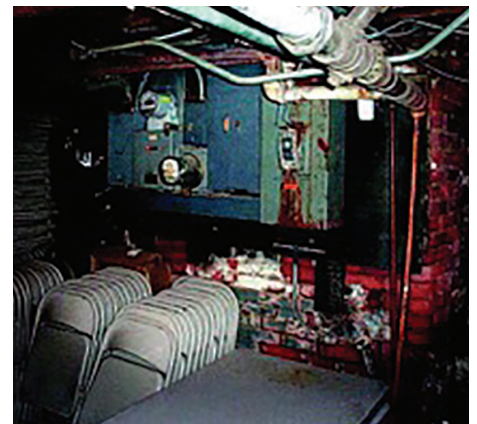
Electrical equipment rooms used for storage create property and liability exposures.
