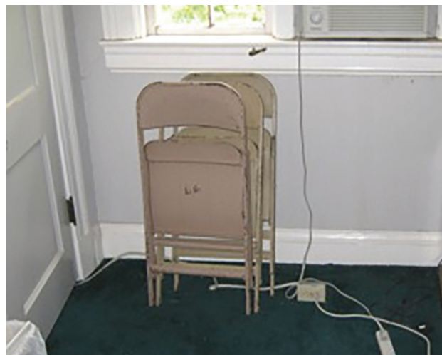
◀ This image shows several wiring hazards; a “homemade” extension cord on the floor that is run under a doorway, which has an outlet installed at the end, that has a power strip plugged into it that is supplying power to a window air conditioning unit. This is a fire just waiting to occur.
