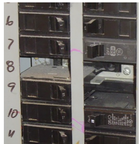
Image above shows open spaces in the electrical panel. Spare clips should be installed in these spaces.
