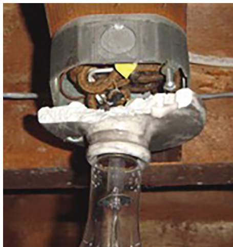
This image shows a broken light fixture. This exposes the wiring to physical damage, dust, dirt and moisture accumulation.
