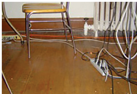
This image shows two power strips that have been plugged into each other, also called daisy chaining. This practice should not be permitted.
