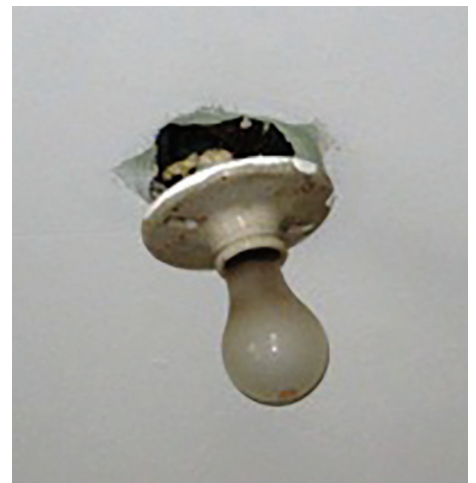
This image shows a light fixture that is unsupported, which puts undue stress on the electrical connections.
