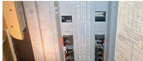
This is a Stab-Lok panel showing the shape and color of Stab-Lok breakers. The handle shape and color are somewhat unique to Stab-Lok breakers.
